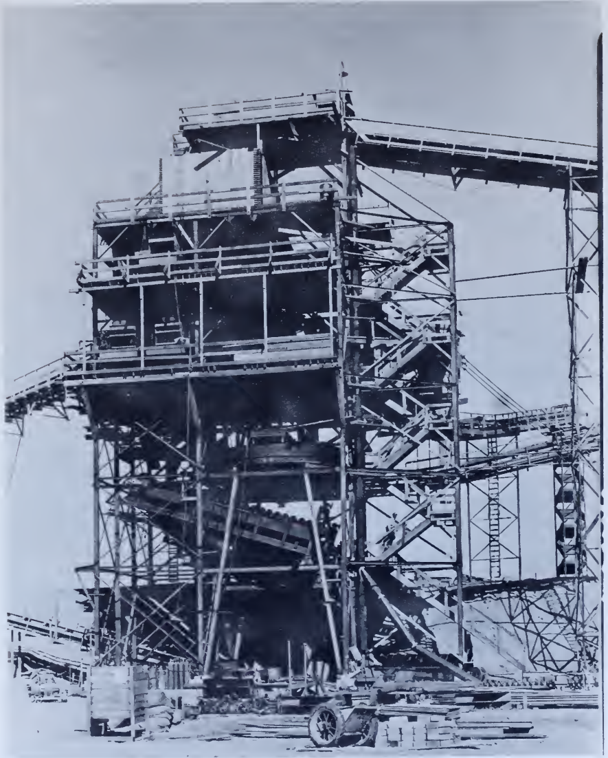
Figure 78.—A well-designed plant used for screening and washing aggregates. PX-D-32059.
